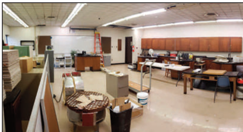
Top, Renovations to the Unmanned Aerial Technology Program's classroom at the West Richland Center are now complete. Above, Work begins on the project last fall.
