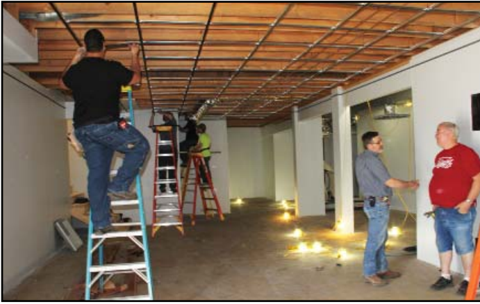
Construction Technology students installed the ceiling grid in the weight room. Adjunct Instructor Larry Barbre shown at right in blue shirt is overseeing the students' work.
