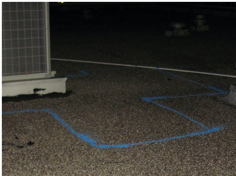
Wet Area #3: The distinct board pattern of wet insulation indicates that the insulation is saturated in this area.
