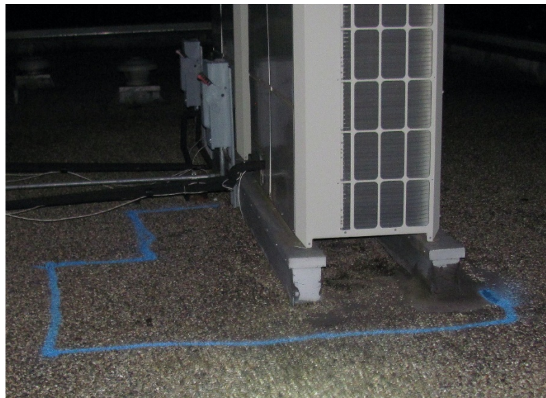
Wet Area #6: Sub-surface moisture was detected around these air handling unit curbs.
