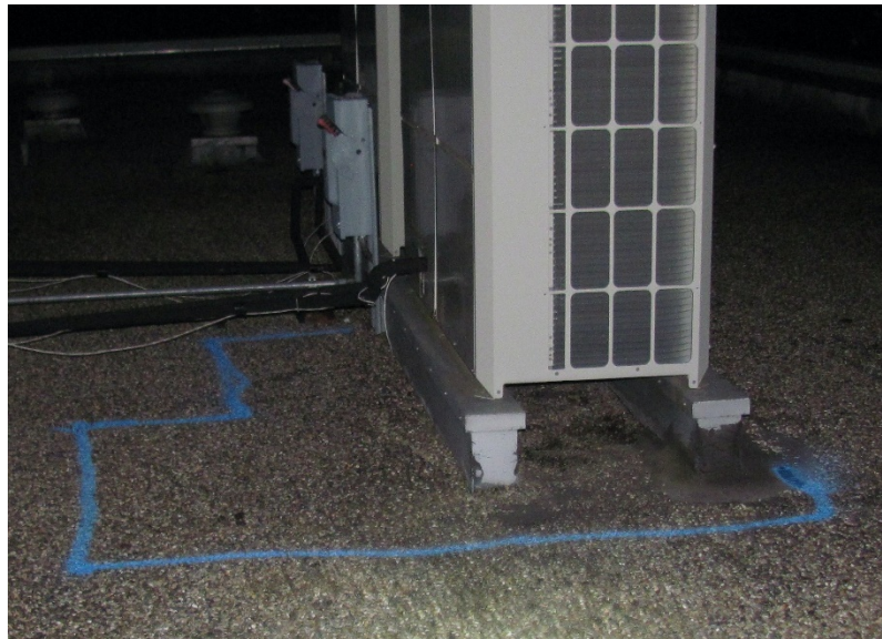
Wet Area #6: Sub-surface moisture was detected around these air handling unit curbs.
