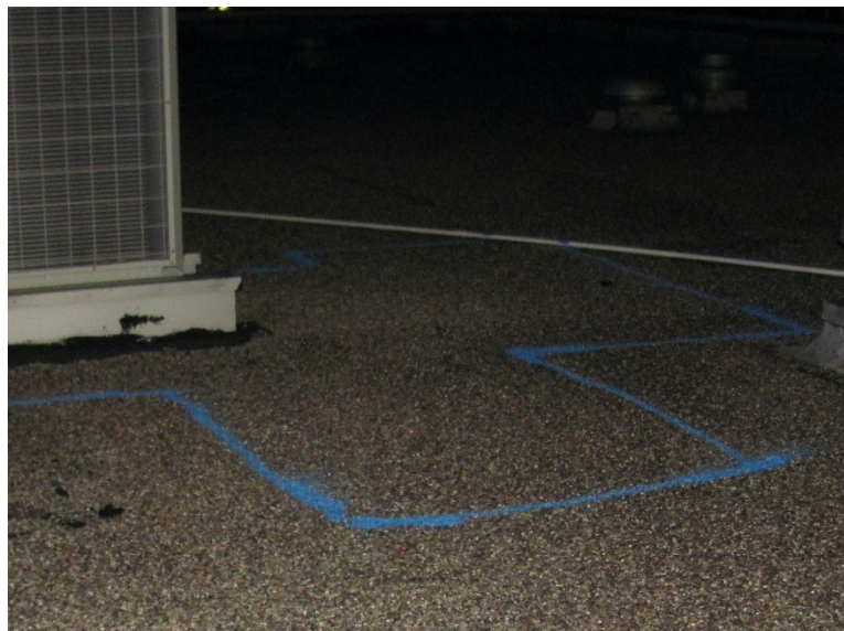
Wet Area #3: The distinct board pattern of wet insulation indicates that the insulation is saturated in this area.
