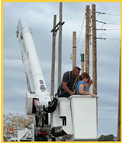
EDS Instructor Dustin Wiggins showing student how to be properly harnessed before operating the bucket truck
