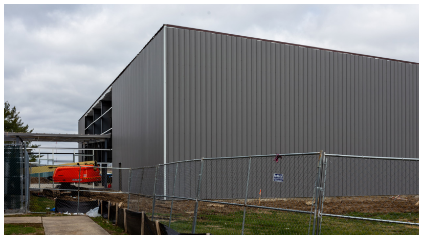
Work continues on the Crawford County Recreation Center. Workers erected the steel frame of the building and then started work on the exterior of the building. The project is expected to be completed this summer with the facility opening to the general public in late summer or early fall.
