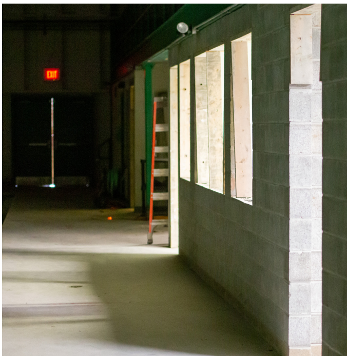
Work continues on the Rowland-Nicholas Natatorium. Rough framing of the rooms is completed.
