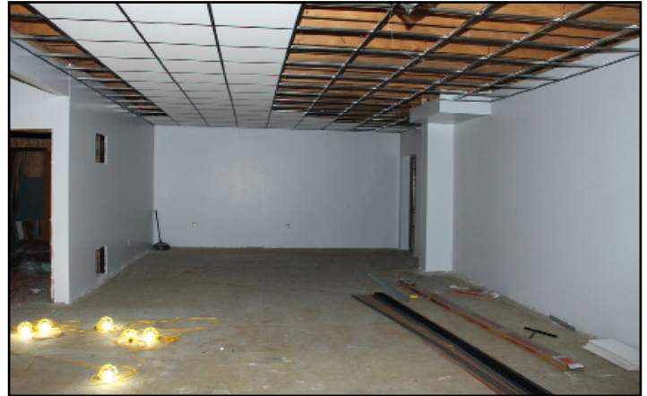
The dry wall is finished and a coat of fresh paint has been applied to the weight room. Ceiling tiles are going in.
