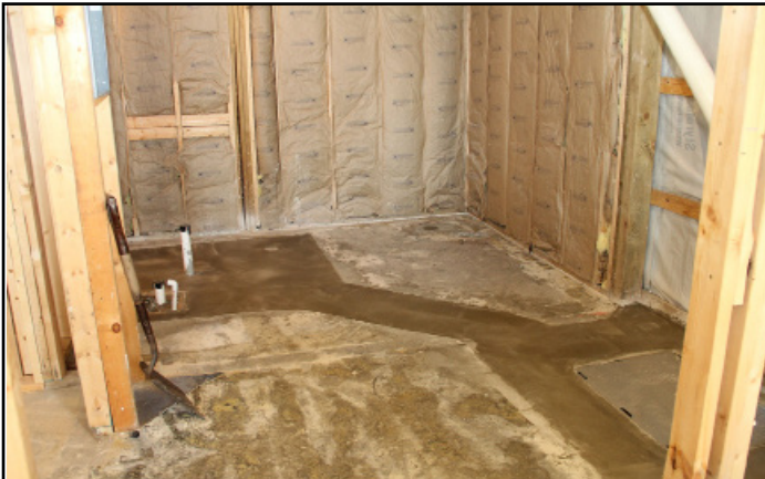
Plumbing has been roughed in and concrete poured in the Bobcat Coffeehouse / student lounge.
