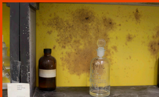
CHEMICAL RUSTING IN STORAGE AREAS
